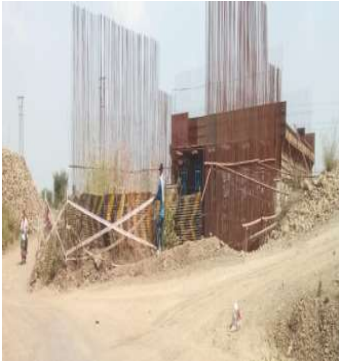
CH. 114+900 HAZARD AREA BARRICADING
