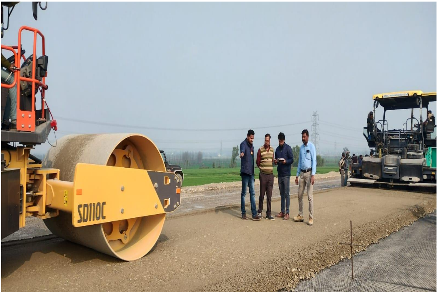
WMM Trial Patch with Triaxial Geogrid under process at ch-19+350. With SPS , SQME, ME sir
