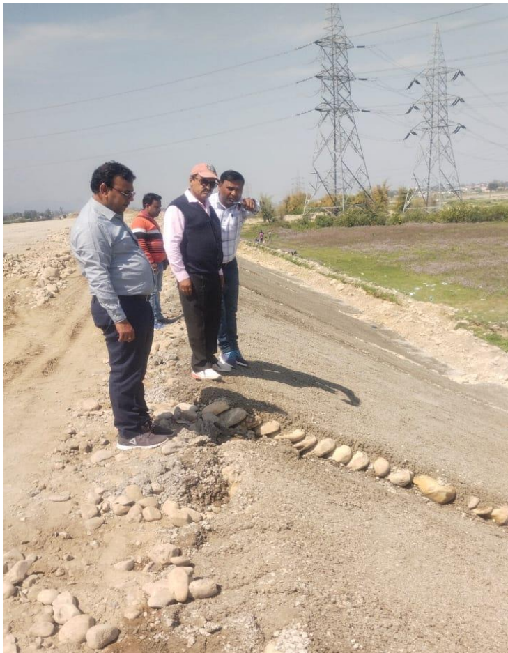
Slope Protection Work Jointly Inspected by RE sir & BE sir along with MKC Team
