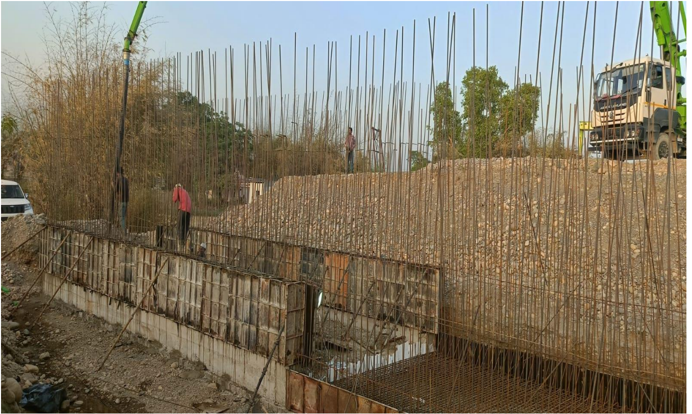
Box Culvert Wall 1st Lift Concrete Pouring Work in Progress at Ch. 27+068
