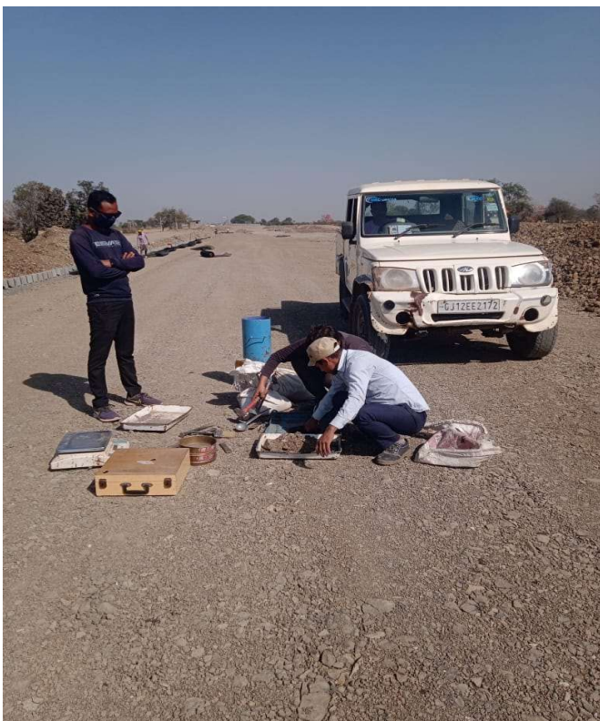
Ch:95+090 to 95+460 Lhs re wall back filling 25th layer (w4) fdd check
