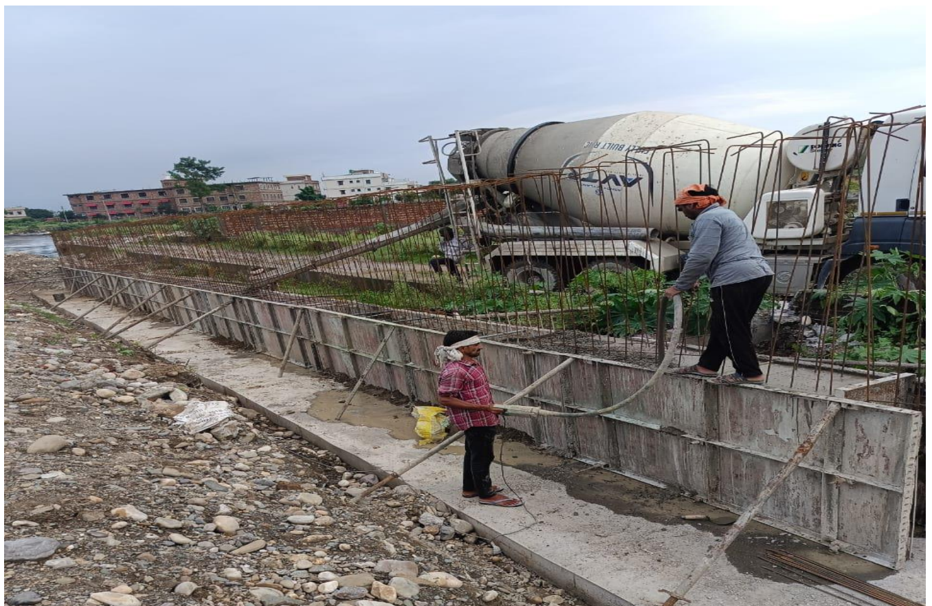
Toe Wall 1st Lift Pouring Work in Progress at Ch. 32+860 to 32+890 RHS
