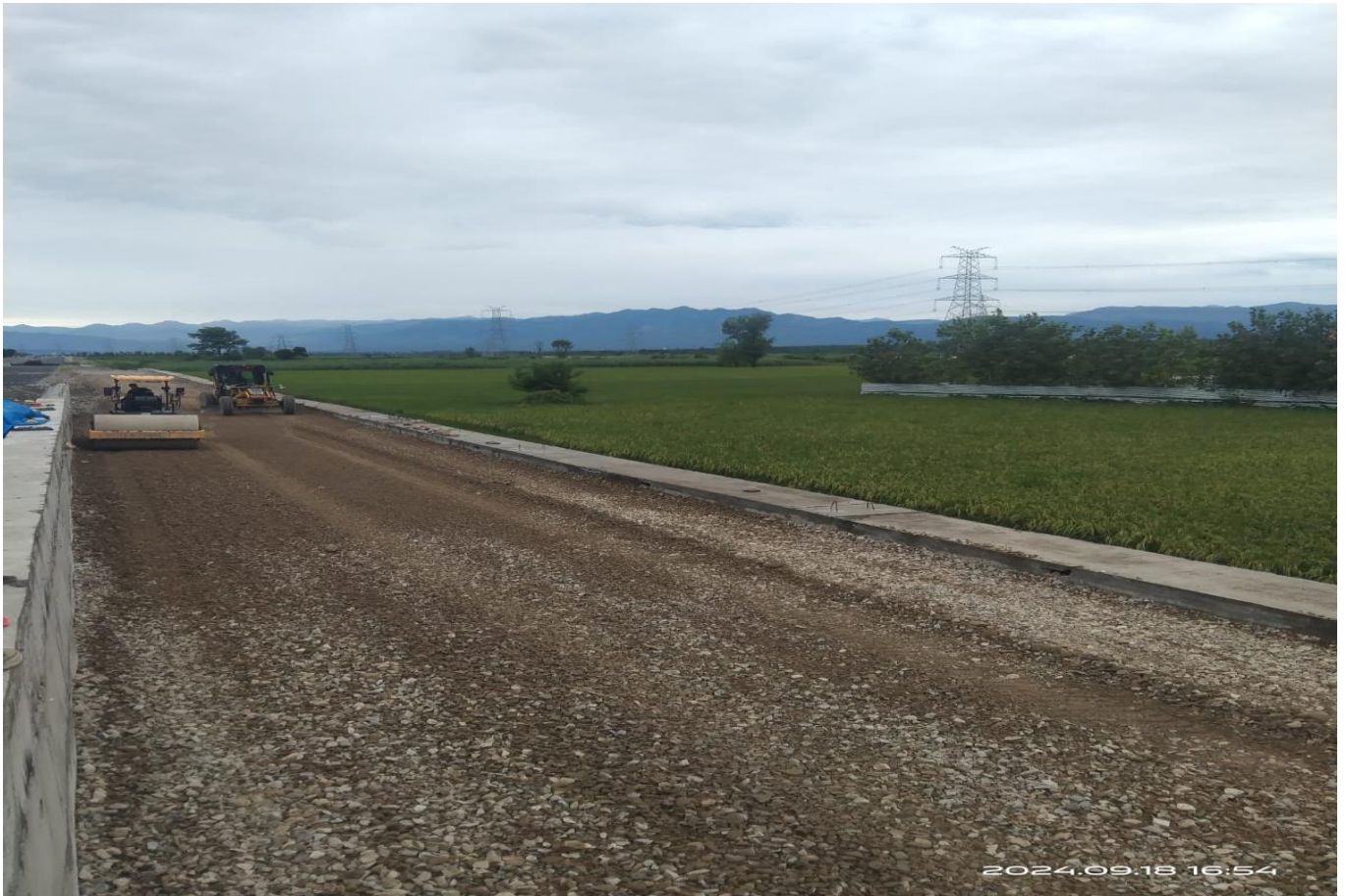
Service Road GSB Top Rolling Work in Progress at Ch. 25+040 to 25+140 LHS
