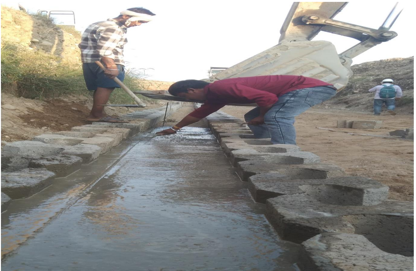
RE Wall Leveling Pad PCC Work in Progress at Ch. 22+740 to 22+800 LHS
