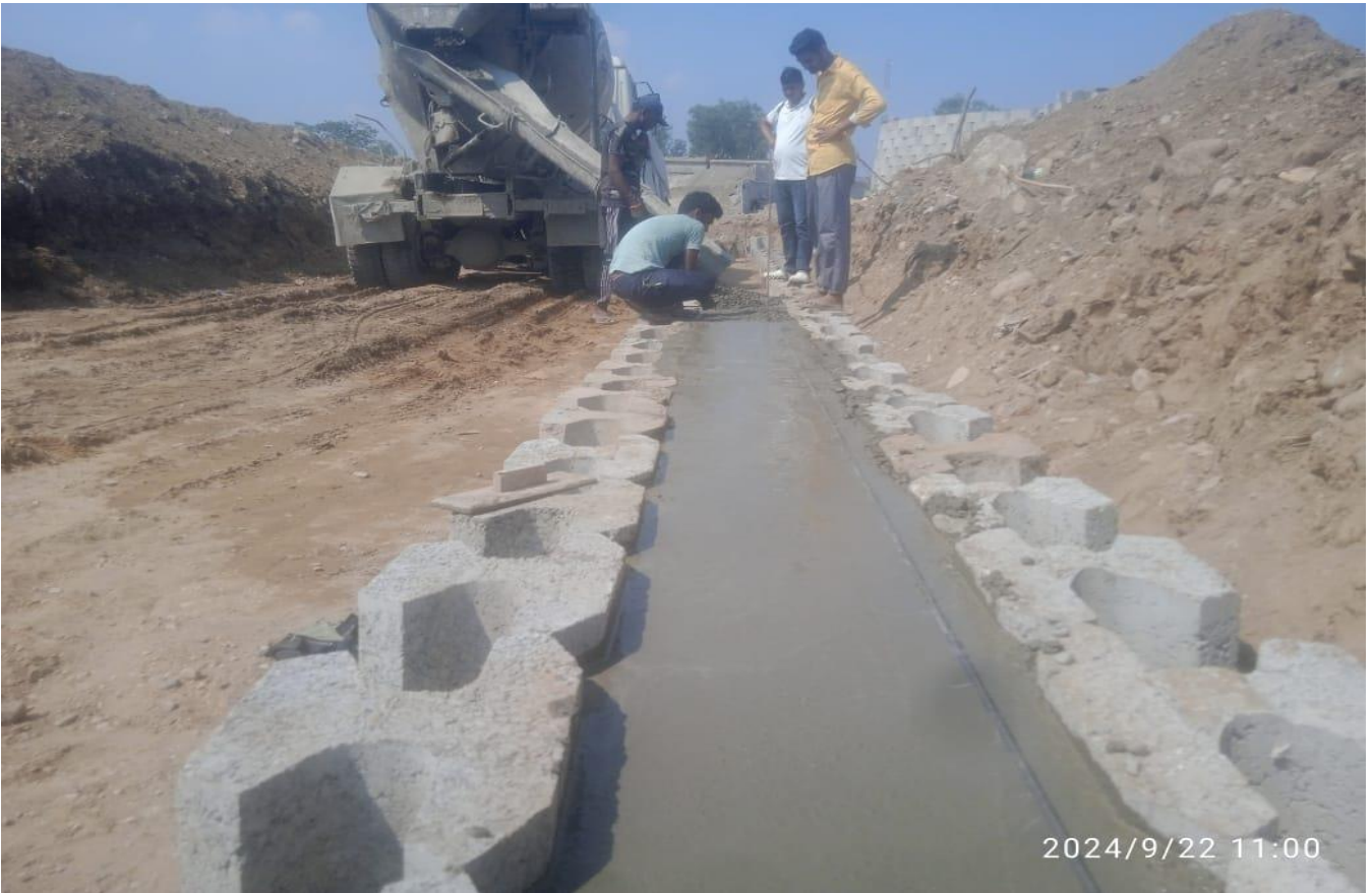
RE Wall Leveling Pad PCC Work in Progress at Ch. 31+800 LHS A2 Side
