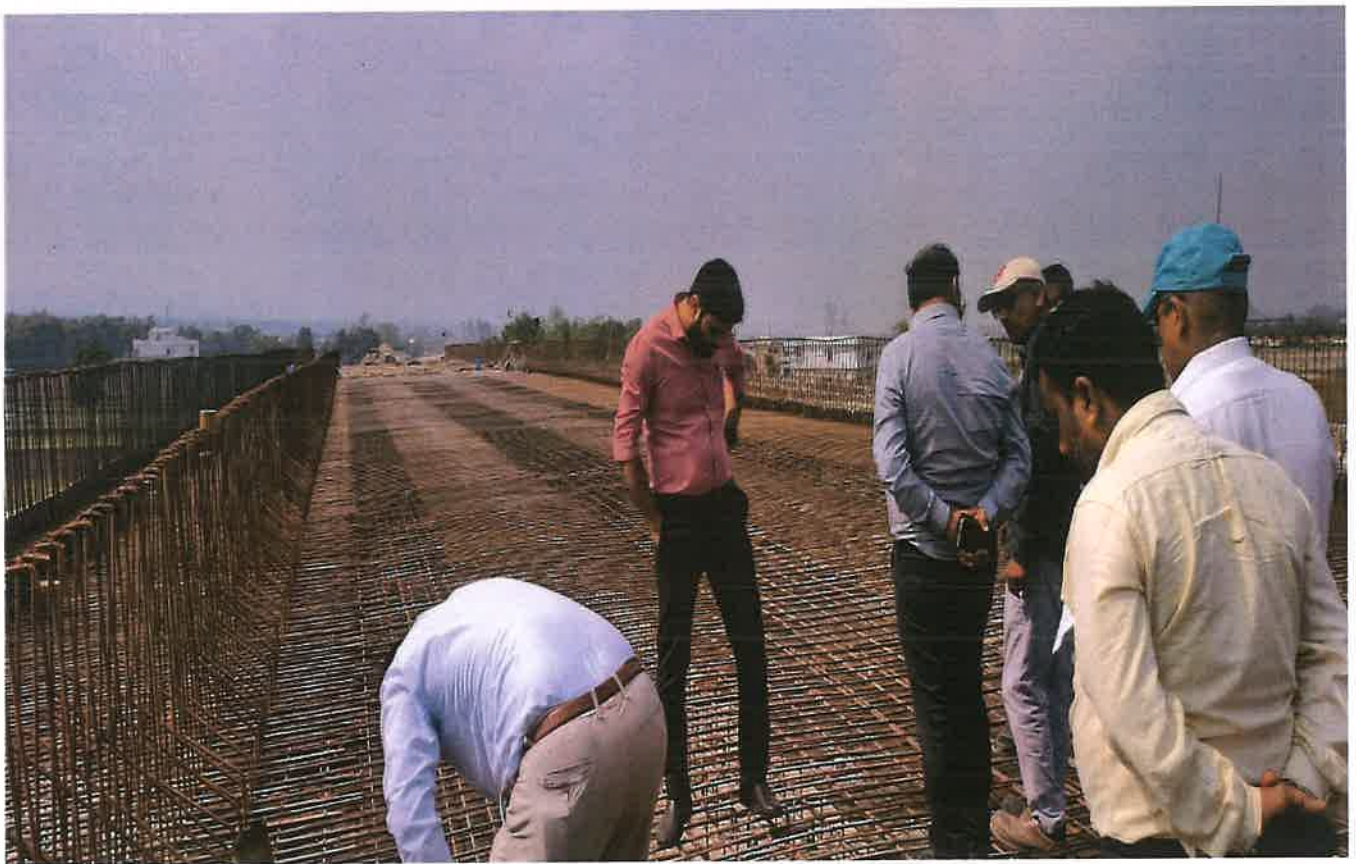
Reinforcement and shuttering checking by Manager Tech , RE and BE at MJB 33+033.
