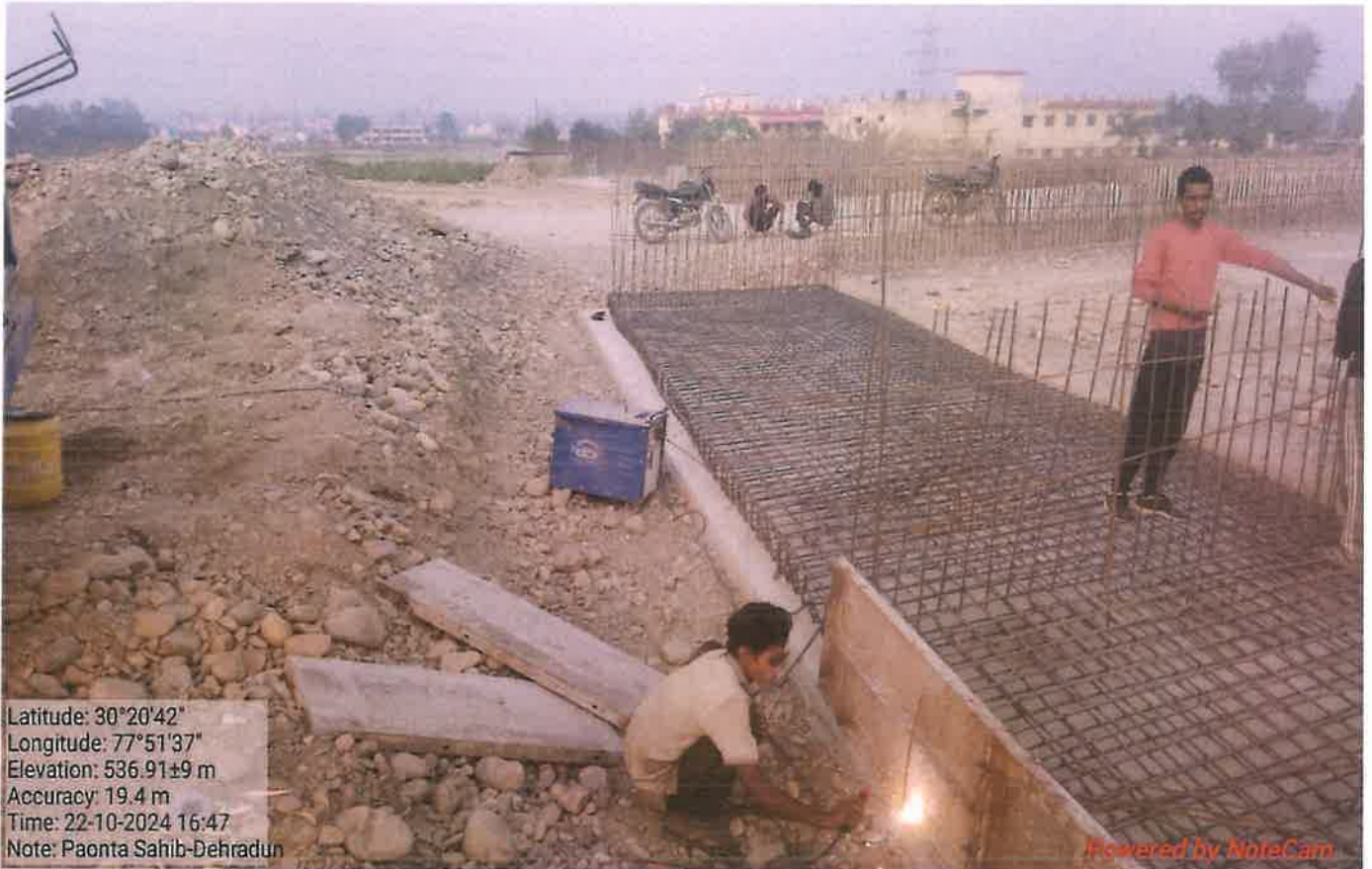
A1 RHS service road approach slab reinforcement binding work in progress at MNB 29+659
