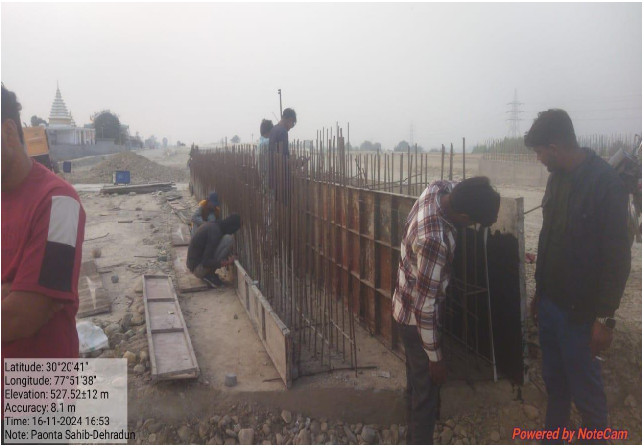
MNB Crash Barrier & Parapet Wall Reinforcement & Shuttering Work in Progress at Ch. 29+659
