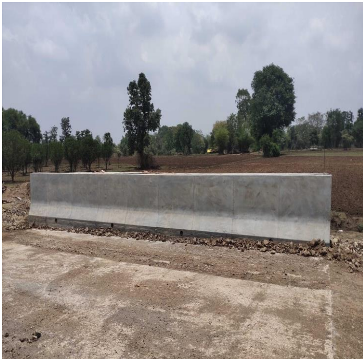
Crash Barrier at Ch- 99+345
