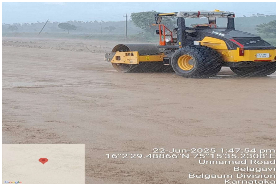
Plate 18 Highway Work Got Hindered due to Heavy Rain at Ch. 81+900
