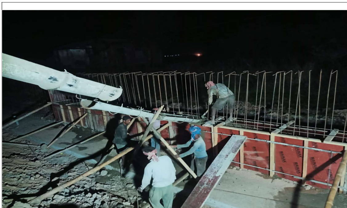
TOE WALL 1ST LIFT CASTING WORK IN PROGRESS AT CH FROM 55+624 TO 55+648(RHS SIDE)
