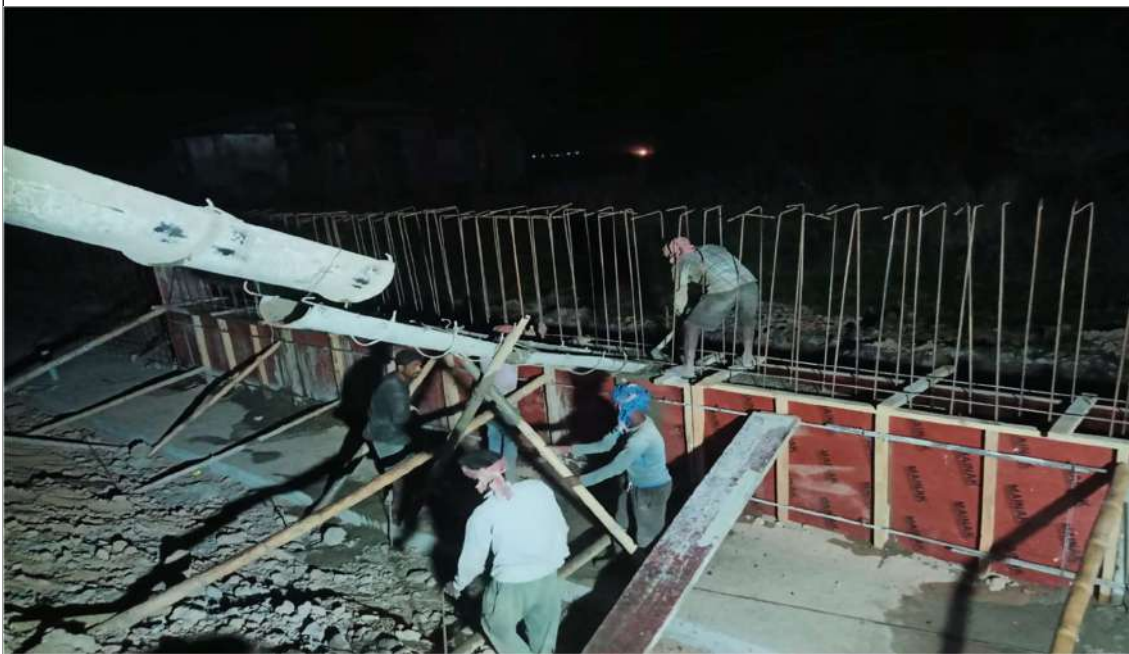
TOE WALL 1ST LIFT CASTING WORK IN PROGRESS AT CH FROM 55+624 TO 55+648(RHS SIDE)
