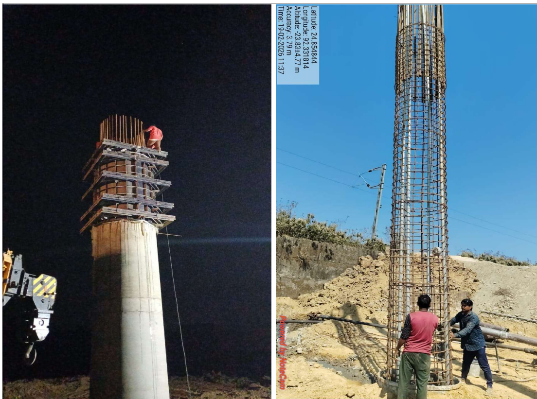
MJB- Pier Shaft Final Lift Concrete in Progress At 5+332 ROB- P1 Pile Cage in Progress At Ch-4+624
