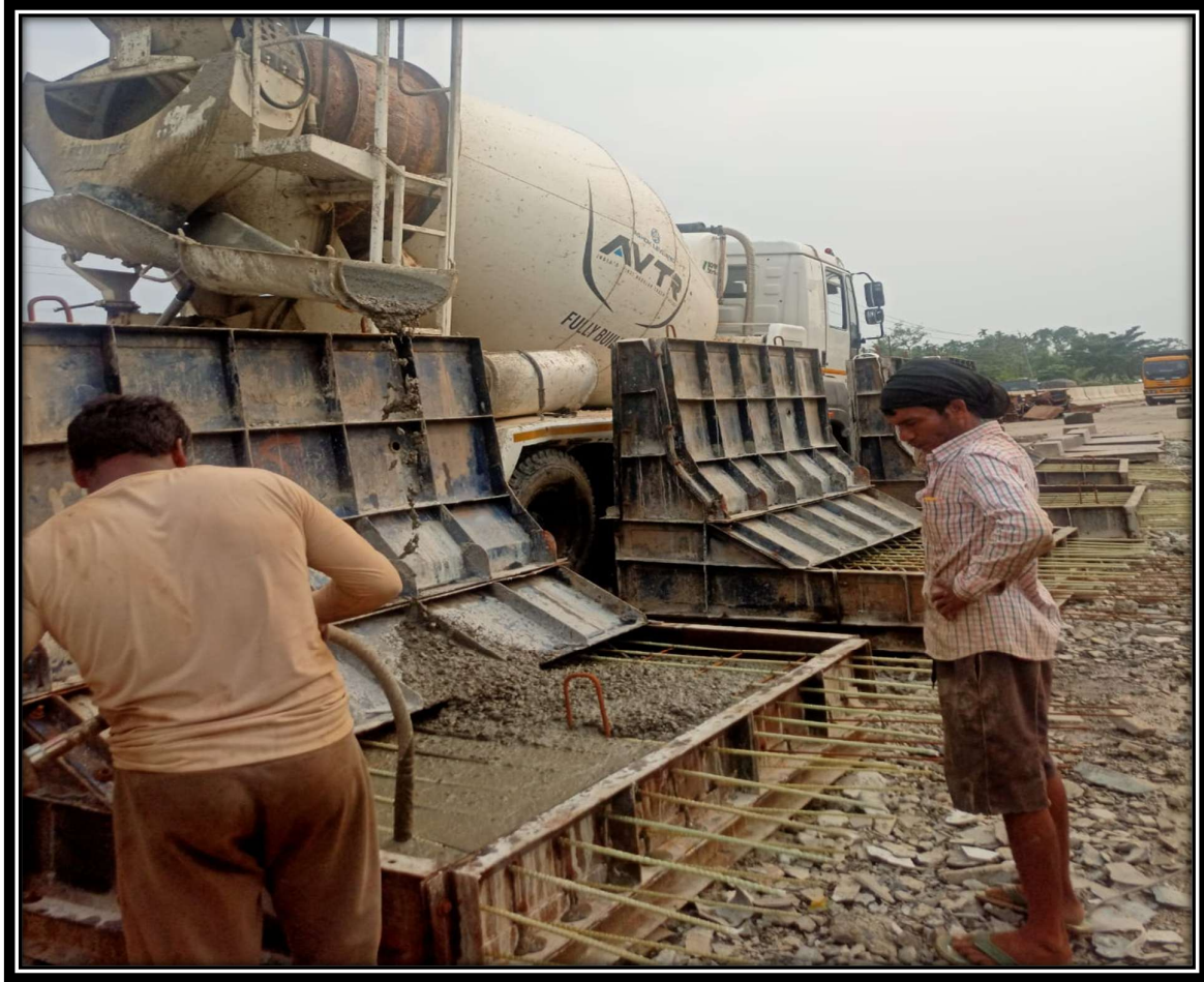
Precast friction slab crash barrier concrete pouring work in progress at toll plaza (casting yard)
